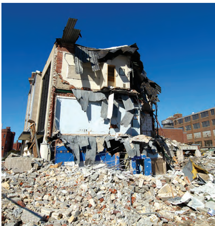
Remnants of the former Worcester Industrial Technical Institute. Demolition should be completed this spring.
